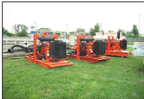
Three Godwin HL5MS Pumping 750gpm on 150' TDH with pressure controls
