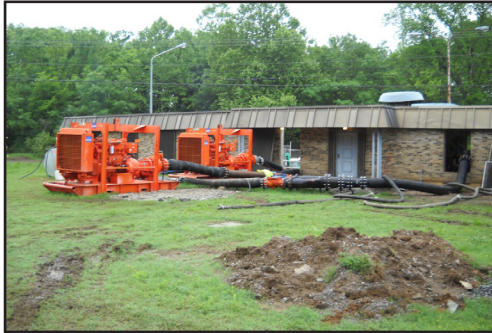
Two Godwin HL250M Pumping 4000gpm each at 250' TDH
