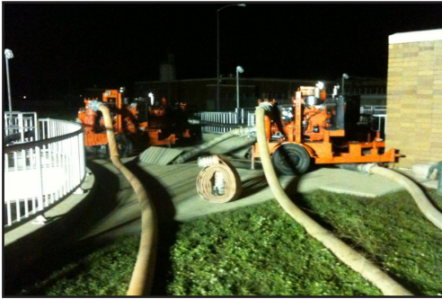
Two Godwin CD150 Pumping 1250GPM each on 50' TDH
