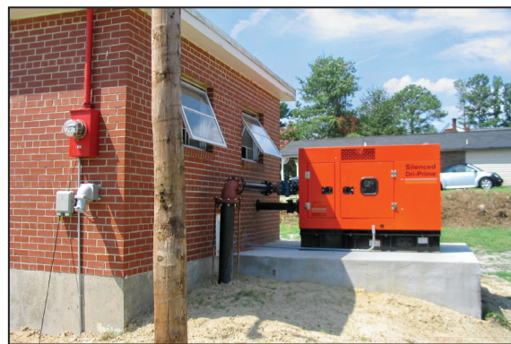
Permanently installed Dri-Prime pump at Edenton, NC.
