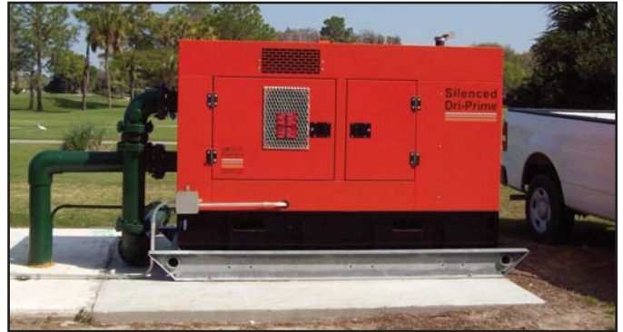
Forty-one Godwin Dri-Prime Backup System (DBS) units have been installed throughout Pasco County, FL, to protect environmentally sensitive areas.
