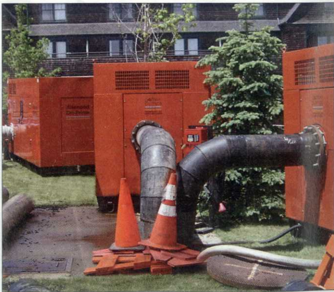
... these temporary backup pumps supplemented the flow during the replacement. Photos: Godwin Pumps.
