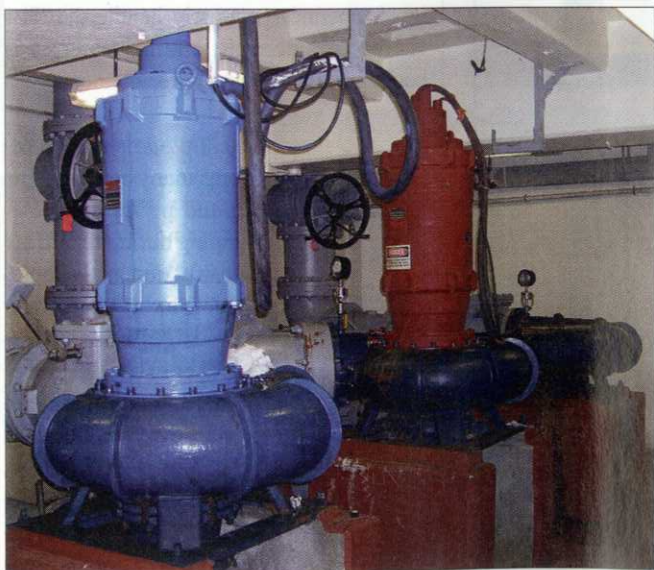
While these electric submersible pumps were being replaced inside the wet well ...
